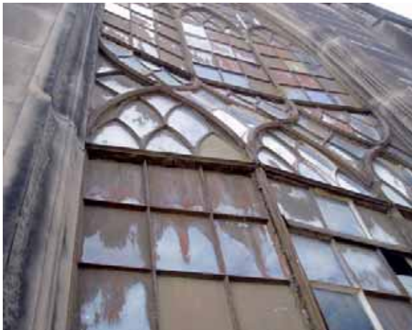
NE window before repair
