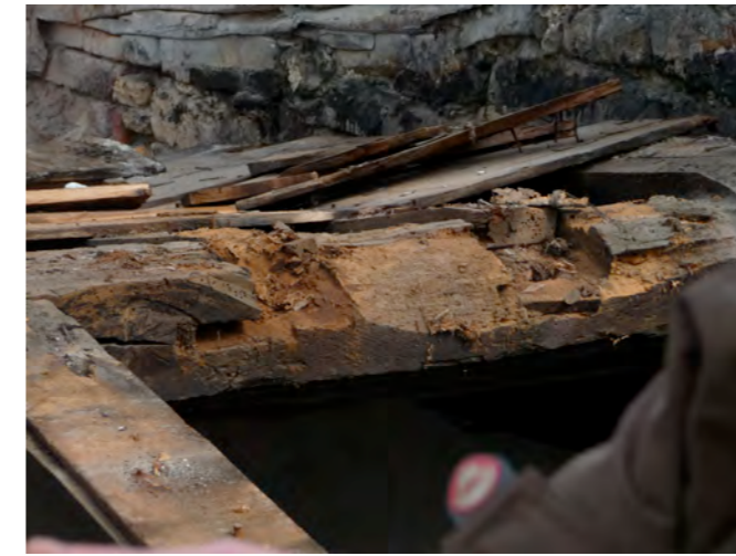
Decay of ridge member.
