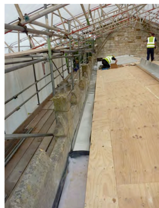
Finished roof prior to laying of stainless steel. The steel work is below the plywood deck.
