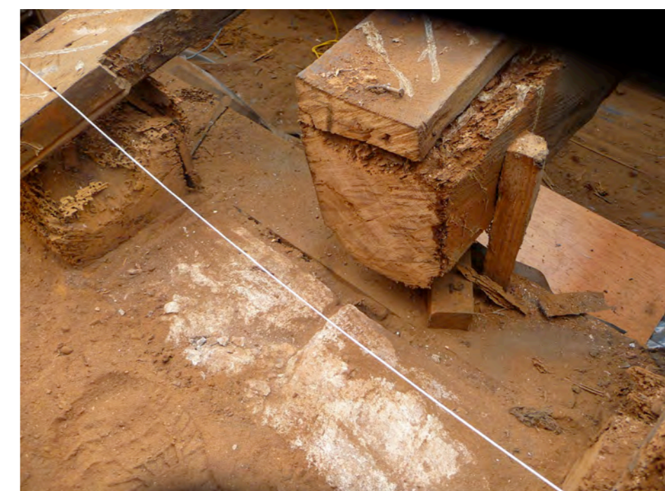
Photograph showing one rafter end following trimming of frass. It falls short of the bearing by 50mm.
