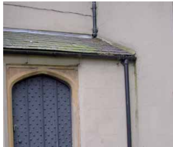
Defective render and cement fillets, overflowing rainwater
