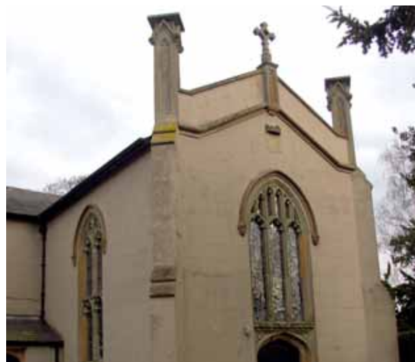
Poor quality renders to west end and truncated pinnacles
